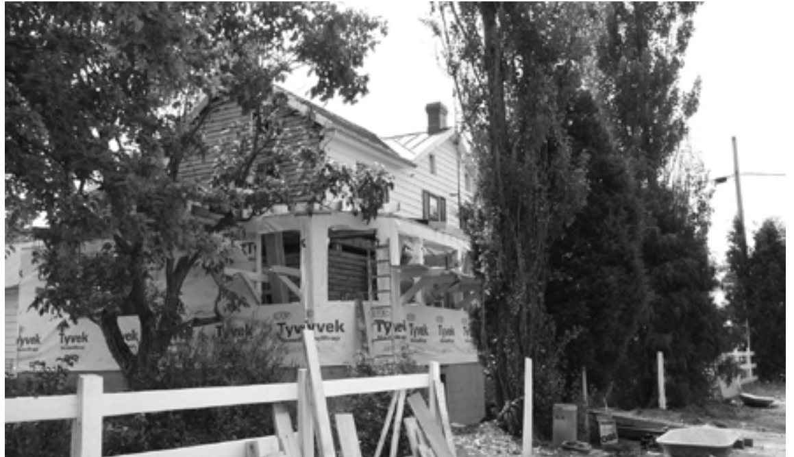
Less than ten days after the permits were issued, the addition was framed and enclosed.
