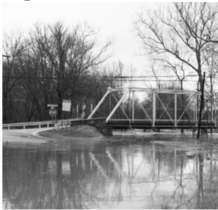
Tom's Creek flooding at Tom's Creek Bridge
