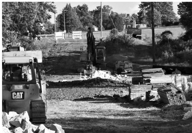
Motters Run Bridge on Motters Station Road is closed while the State Highway Administration constructs a replacement.
