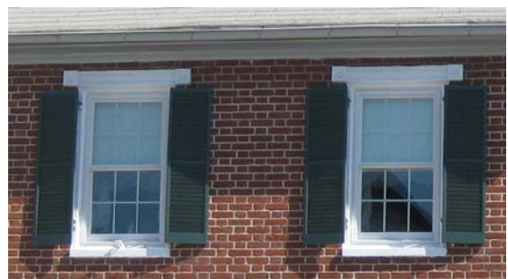
Operable shutters Source: Keith Suerdieck
